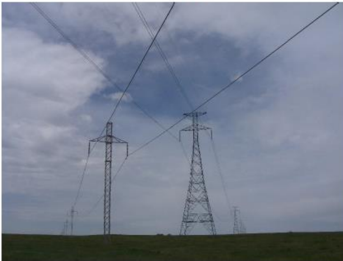
Transmission tower for a HVDC line
