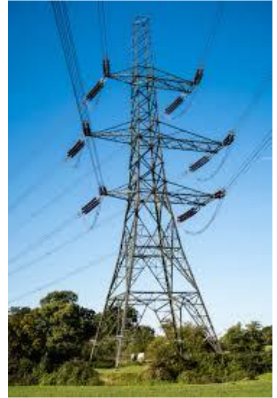
Dead-End Transmission Tower
