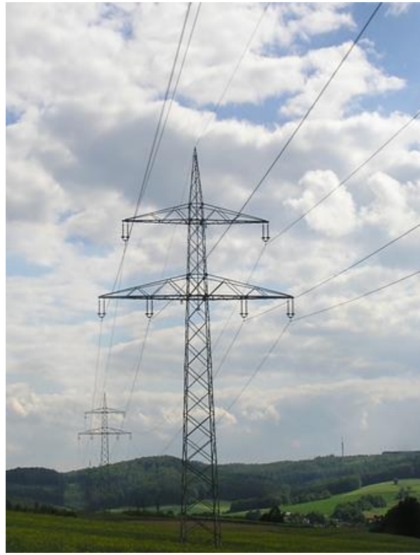
Suspension Transmission Tower
