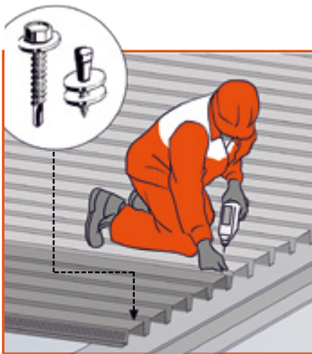
14 - Fix profiles sheets on supports and stitch them among each other (2 fixings per profile sheet and per end support)
