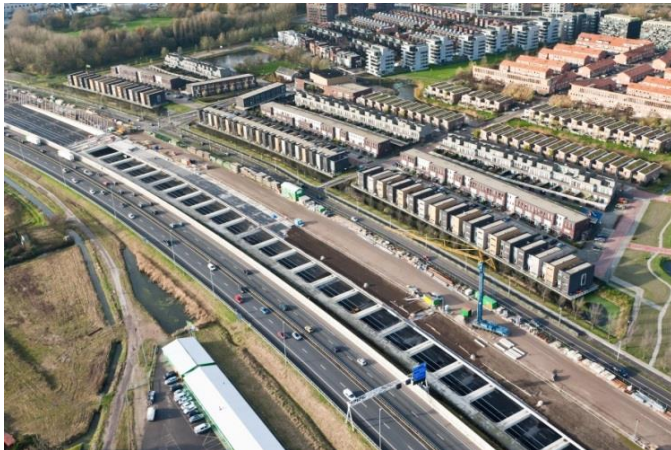
Figure 43 - Overview of the old motorway and new motorway under construction (image source www.beeldbank.rws.nl ).
