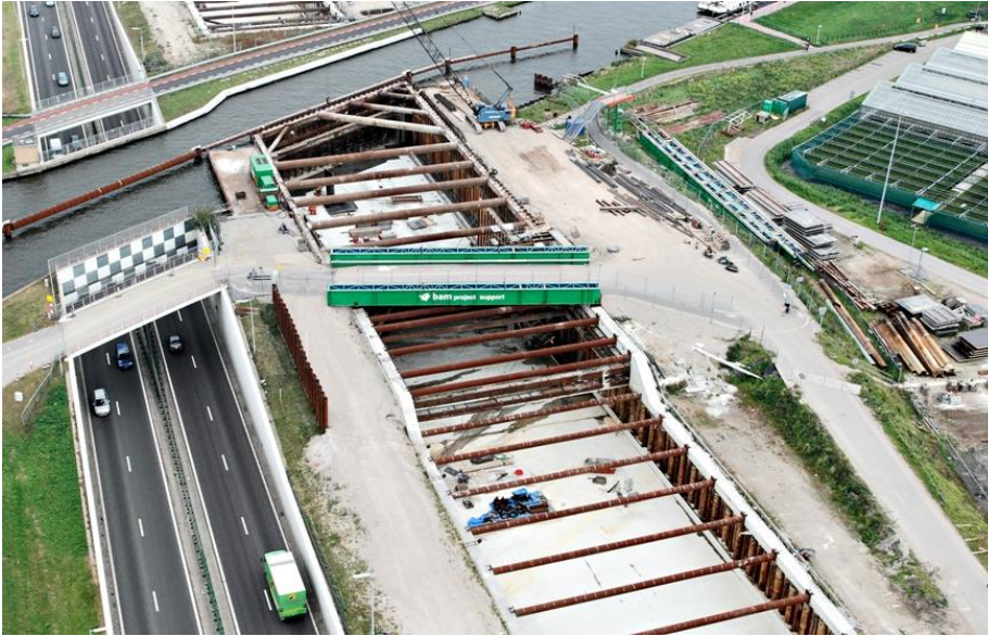
Figure 10 - A4 Ringvaart Aquaduct (highway between The Hague and Amsterdam; the Ringvaart is the canal around the Haarlemmermeer polder, where the airport Schiphol is situated)
